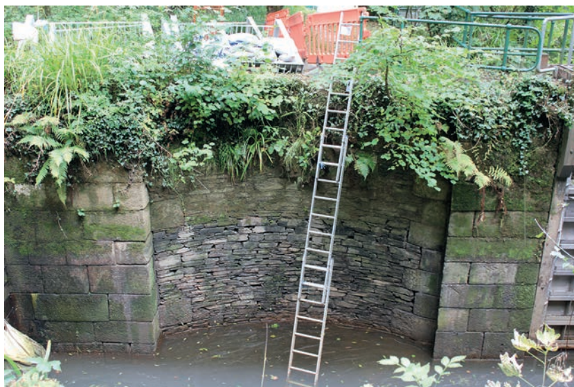
The northern lock on the Tamar Canal during repair work. (Photograph: AC archaeology.)
