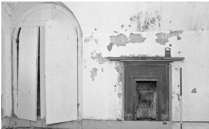
Fig 14 Room F4 showing fireplace and cupboard containing blocked door. Scale 1m. (Photograph: Gary Young.)
