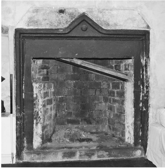
Fig 6 A sixteenth- or early seventeenth-century fireplace in the north room of the central range.
