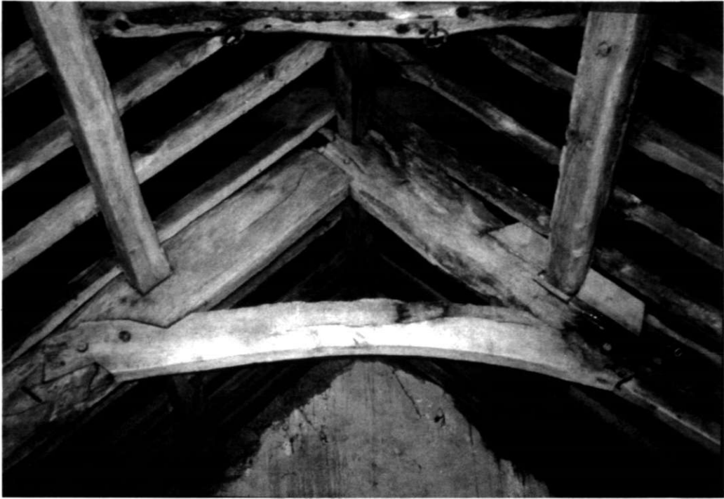
Fig 6 Seventeenth-century roof structure with lapped and dovetailed (or fishtailed) collars to the trusses, over the chamber at the lower end of the house (photo by Eric Berry)
