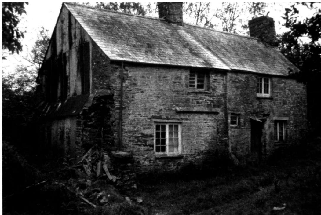
Fig 11 Halbathick as found, prior to renovation and re-instatement of the through-passage and the lower end. The 16th-century oak screen of the original passage survives hidden and protected by corrugated iron (photo by Eric Berry)
