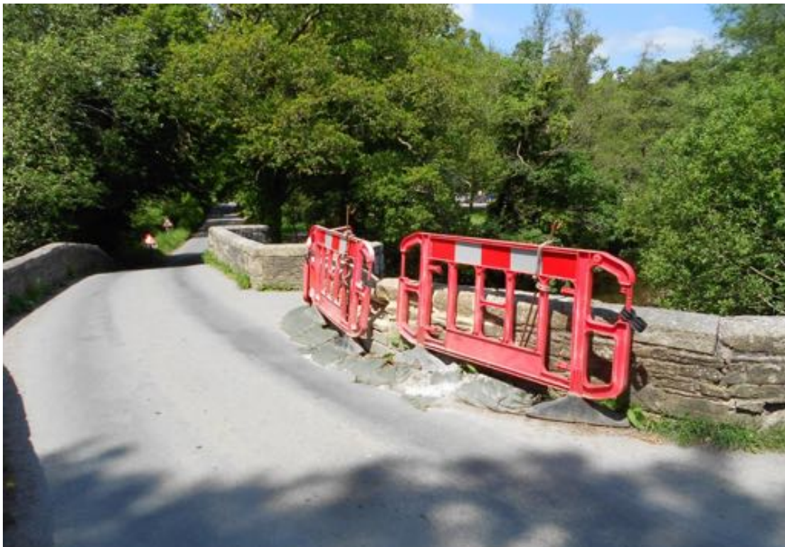
Respryn Bridge is frequently the victim of damage from vehicles, usually accidental.
