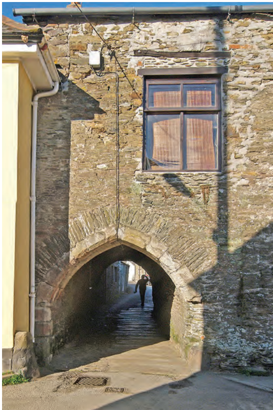
Fig 29 Duchy Palace, Lostwithiel. This almost complete c 1300 doorway spans the river Cober, the base of the doorway infilled but the head of the doorway retaining original dressed Pentewan stone. (Photograph: Eric Berry.)
