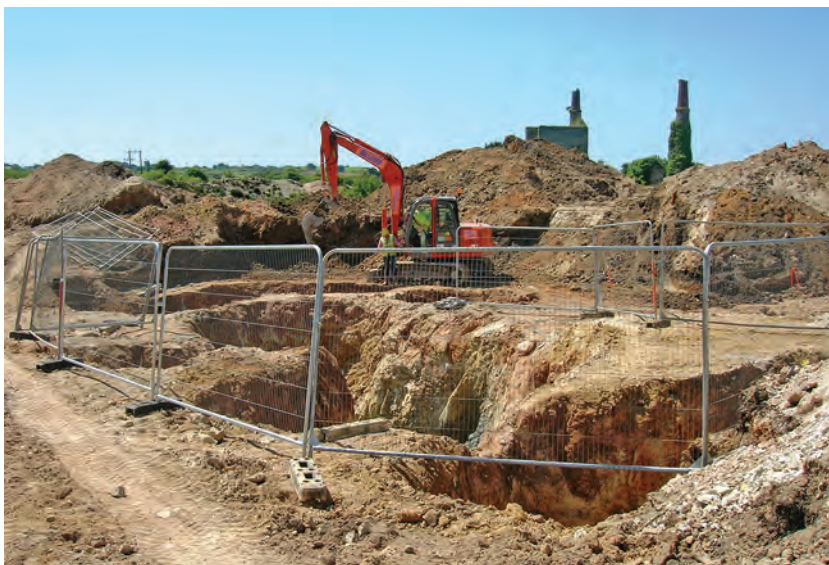
Fig 2 Investigation of outcrop shafts at Hallenbeagle, looking north west towards the two surviving engine houses on the site. (Photograph: Cornwall Archaeological Unit.)
