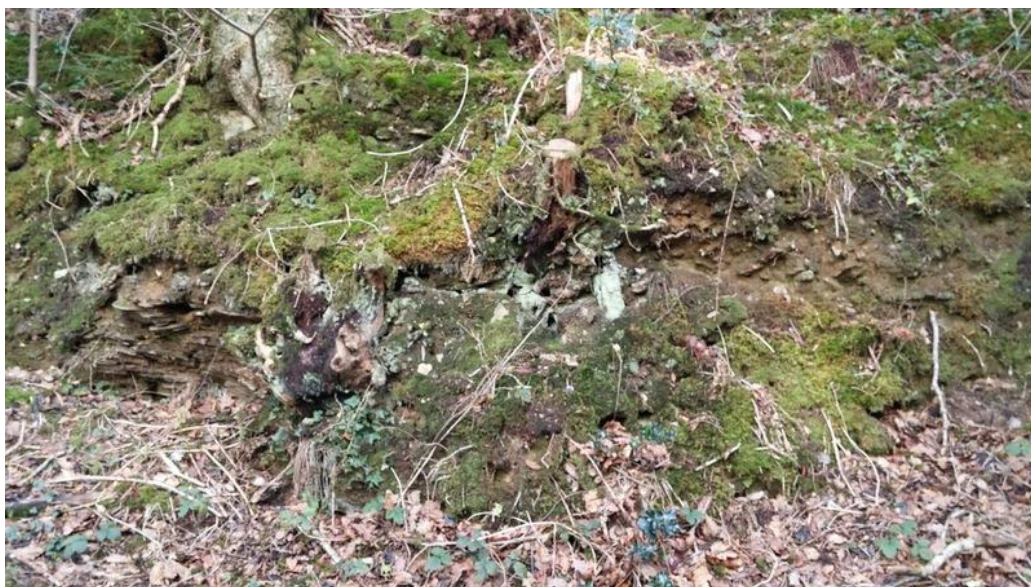
SM 32591 Bishop's Wood hillfort, erosion of section of south rampart due to weathering and root growth.
