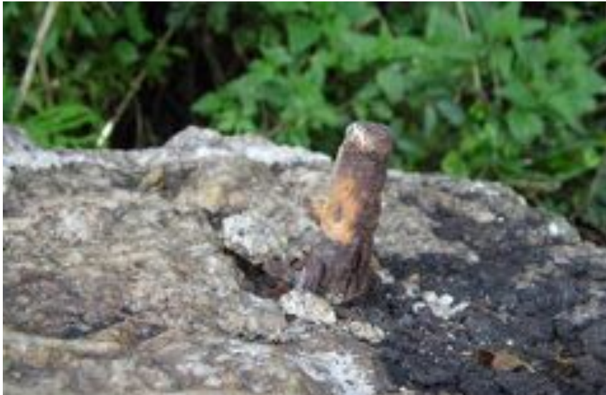
The corroding pin at the top of the cross shaft
